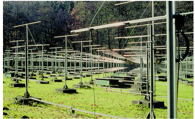
Figure 5. SOUSY antenna array near Bad Lauterberg in the Harz mountains (Source: MPAe).
